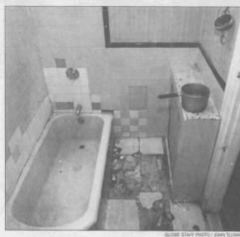
A wall light hangs from exposed wires in a common bathroom with no hot water on the first floor at 30 Morland St. in Roxbury. This photo was taken with a flash because the bathroom light was not working.
